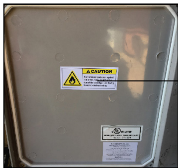
INSIDE OF ELECTRICAL BOX
